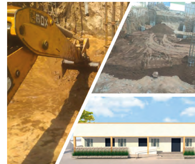
In the Figure: Karur Round Table 138 project for the construction of school buildings in India
